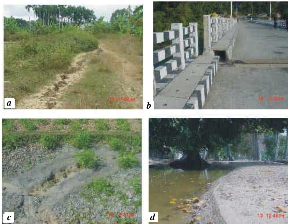
Figure 6. a , North-south trending ground fissures formed near Diglipur. b , E–W shift observed in the span of Panighat bridge near Diglipur. c , Sand blows formed due to ground shaking at Diglipur; the crater shown is about 30 cm in diameter. d , Tsunami deposits about 15–20 cm near Munda Pahar beach.
